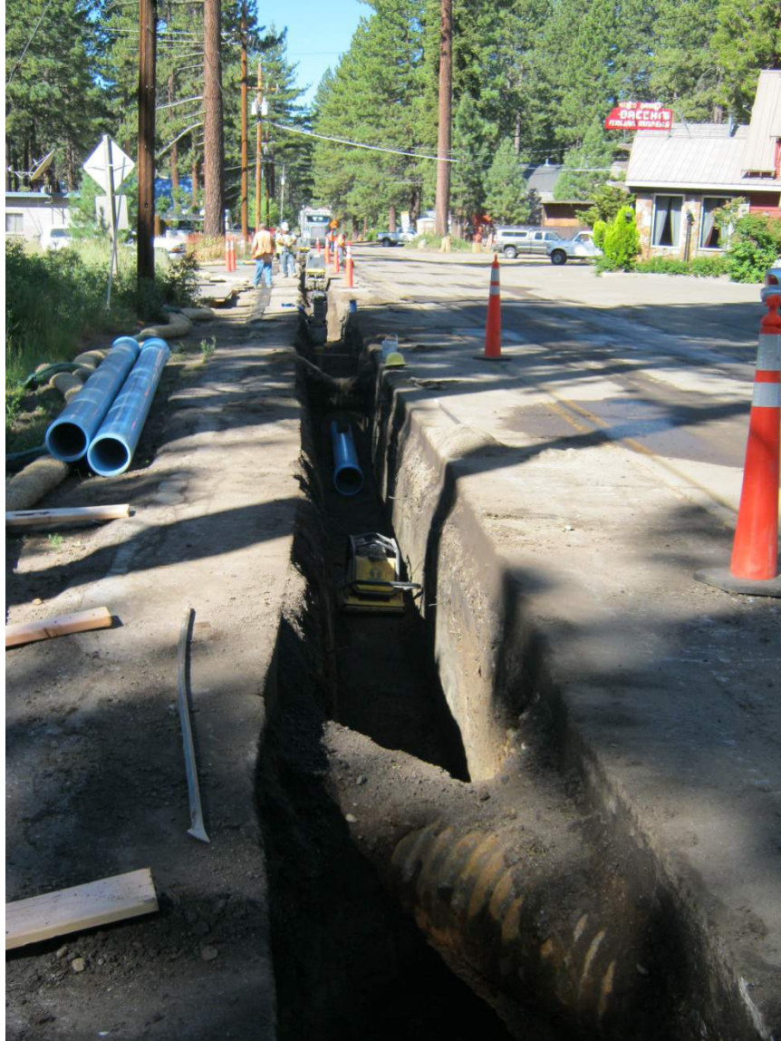
Lake Forest Water System Replacement Project (Lake Forest Road, corner of Aspen)
